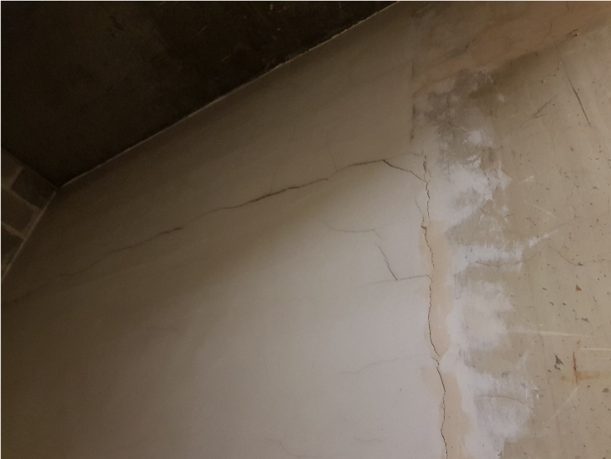
Figure 27: Fire Escape Cracking
