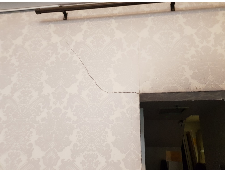
Figure 26: Diagonal Cracking in Tea Room Lintel
