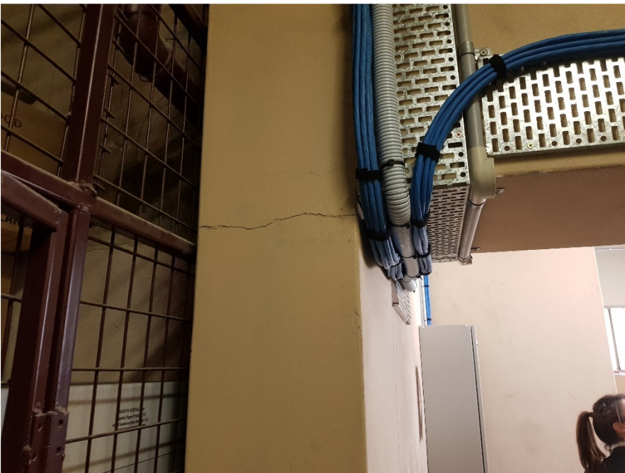
Figure 24: Horizontal Crack in Column
