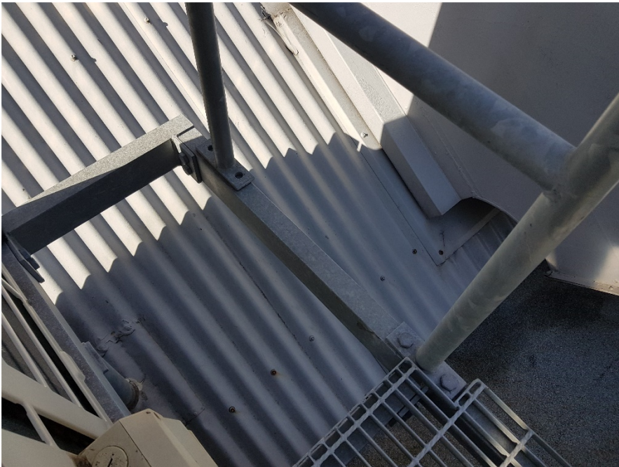
Figure 12: Missing Bolts on Balustrade South End
