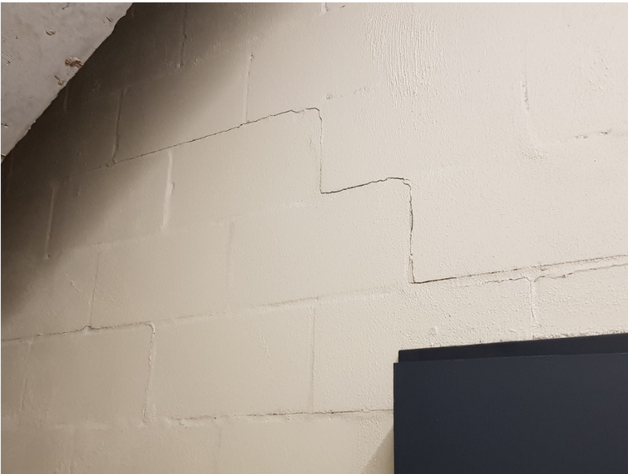
Figure 28: Diagonal Cracking Above Fire Escape Door Opening
