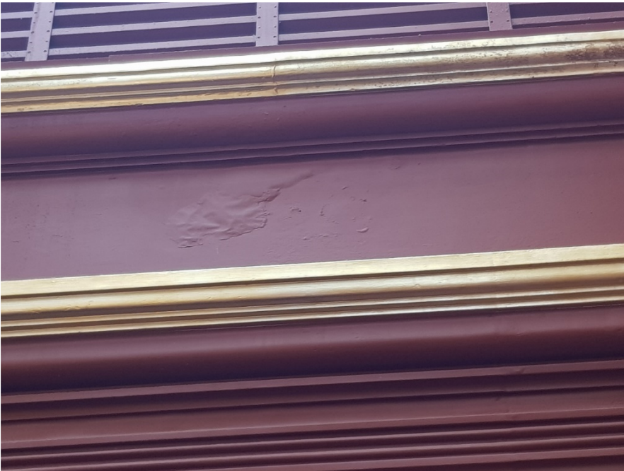
Figure 30: Signs of Water Ingress On Tea Room Entrance Roof
